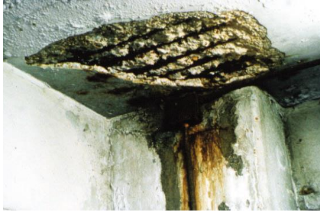
Figure 2-1: Reinforcement corrosion (PCA, 2002)
